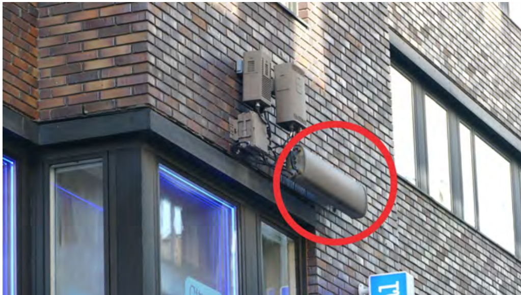
Figure 6: Low positioned base stations at Drottninggatan, Stockholm, Sweden
